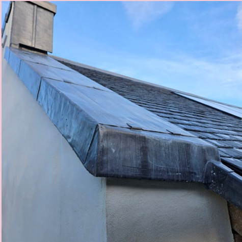
Slating has completed with leadwork and rainwater goods largely complete and already making a significant visual difference.
