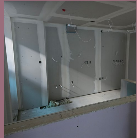
Flats are starting to come together with partitions complete, first fix plumbing & electrics installed. Kitchens will be installed in the next few weeks.
