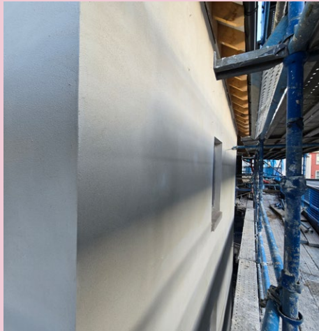
The final render coat has a subtle, machine-finished texture which will be over-coated with a special lime-compatible paint (in white)
