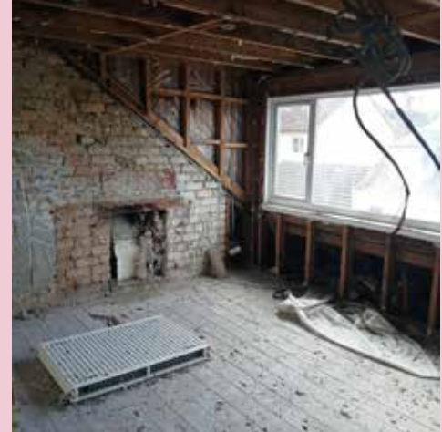
Some areas within the properties are already partially stripped.
