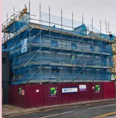
Scaffold/Hoarding at our King's Arms site in Irvine - arrangement likely to be less extensive at Nelson, but safety is always paramount
