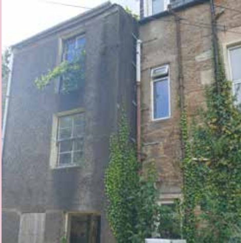
Image structurally compromised extension to be removed Below: garden to rear of property will be cleared
