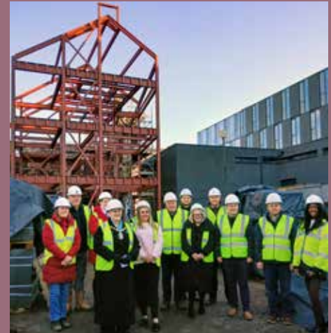
Provost Anthea Dickson at the King's Arms site with Irvine West Councillors Shaun Macaulay, Scott Gallacher and Chloe Robertson; Council officials and staff and representatives from McLaughlin Construction.
